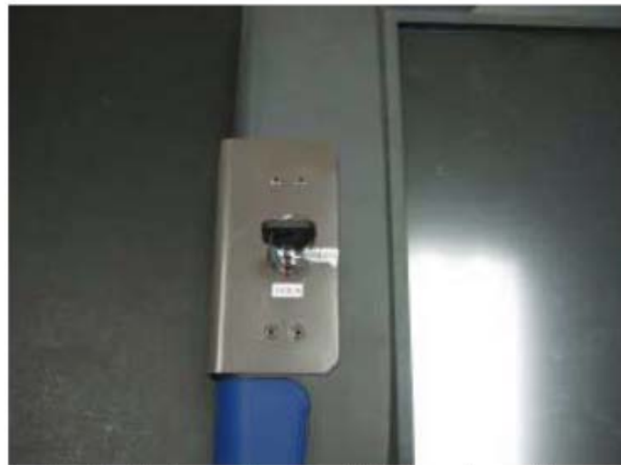
Figure 8.3 – Showing PEB slot covered with lockable metal PEB well cover.
